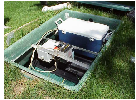
Figure 5: Ecoflo ® Coco Filter Effluent Sampler installed
