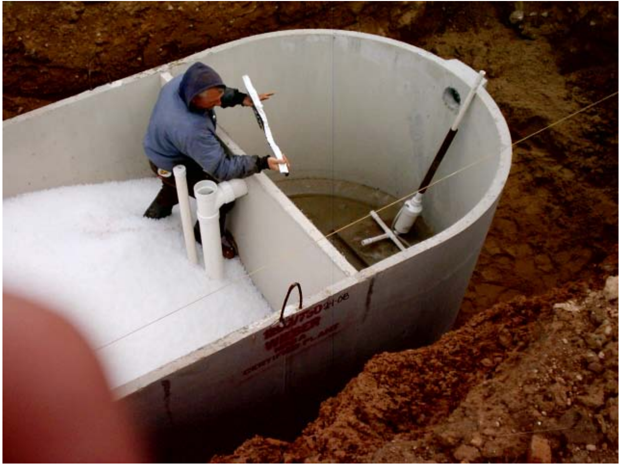
Figure 4 SMART-Treat aerobic reactor/biosolids clarifier with vertical air distribution pipe and carrier element retention screen exposed. The 2 nd compartment also shows the waste biosolids removal pump.
