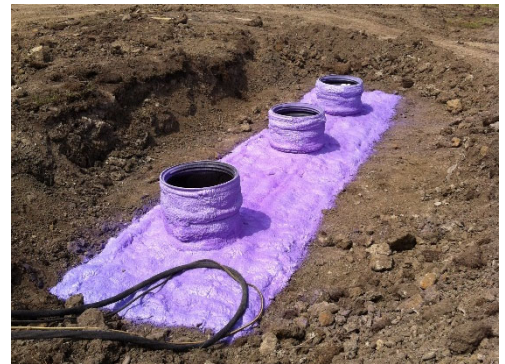
Septic tank with insulation
